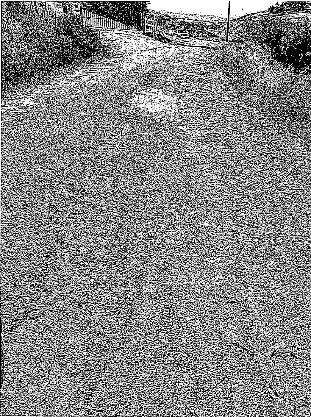
Photo 11: Presidio Way, Chip Seal/Patch Deterioration and Cracking within Wheel Path
