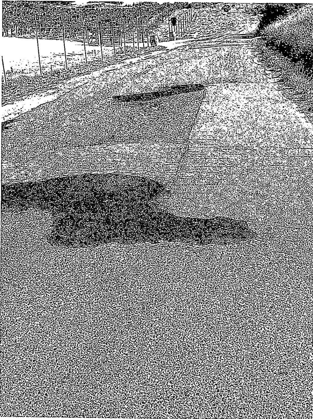
Photo 14: Independence Ranch Place, Patch Deterioration and Cracking in Wheel Path
