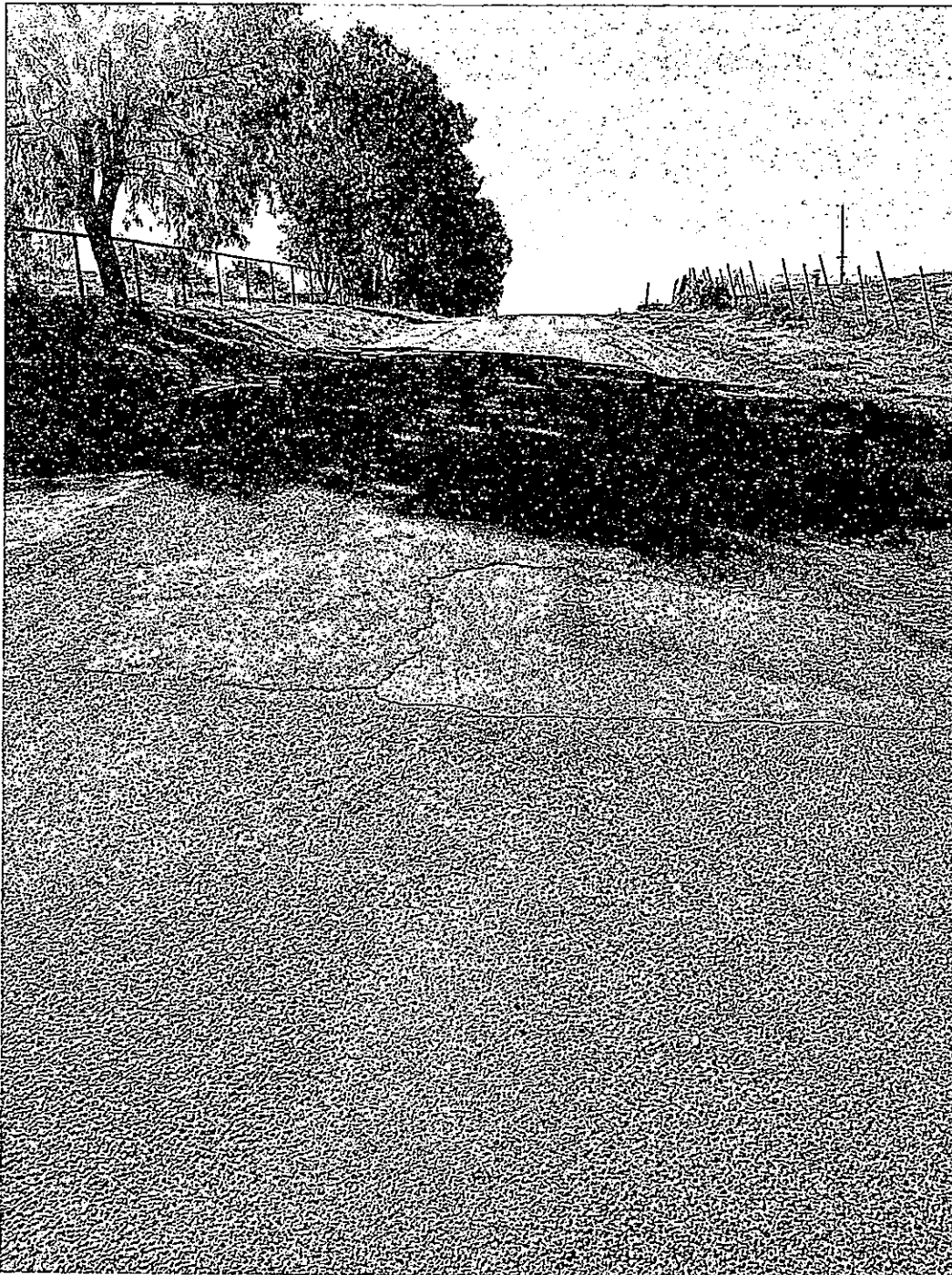
Photo 10: Rancho Lomas Way, Chip Seal and Patch Deterioration
