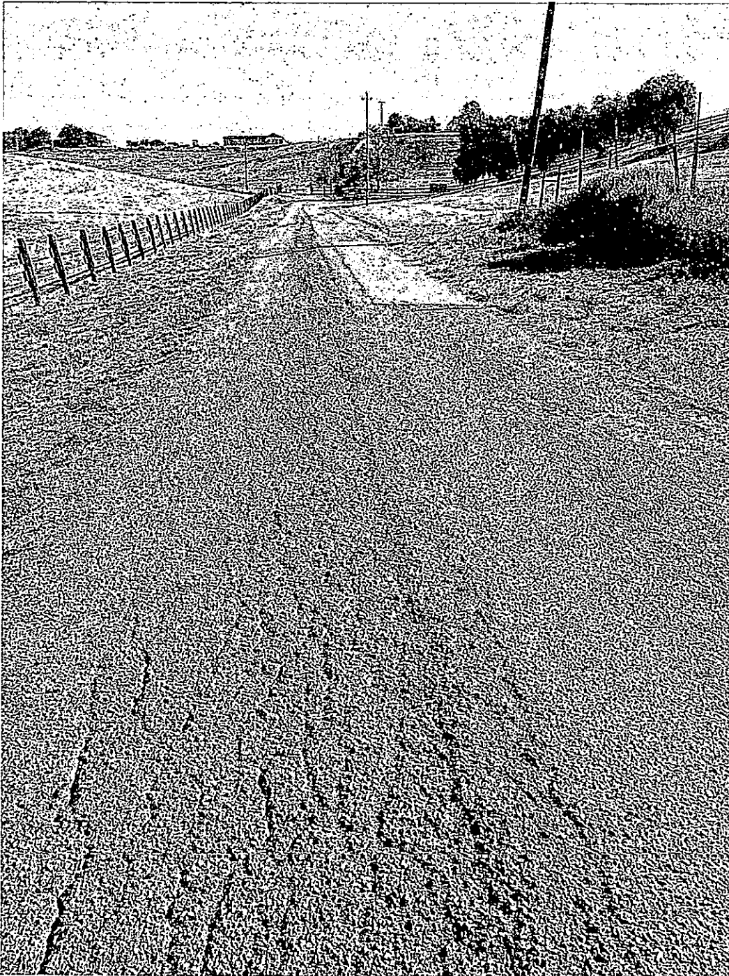
Photo 6: Independence Ranch Place, Cracking within Wheel Path and Pothole Patch
