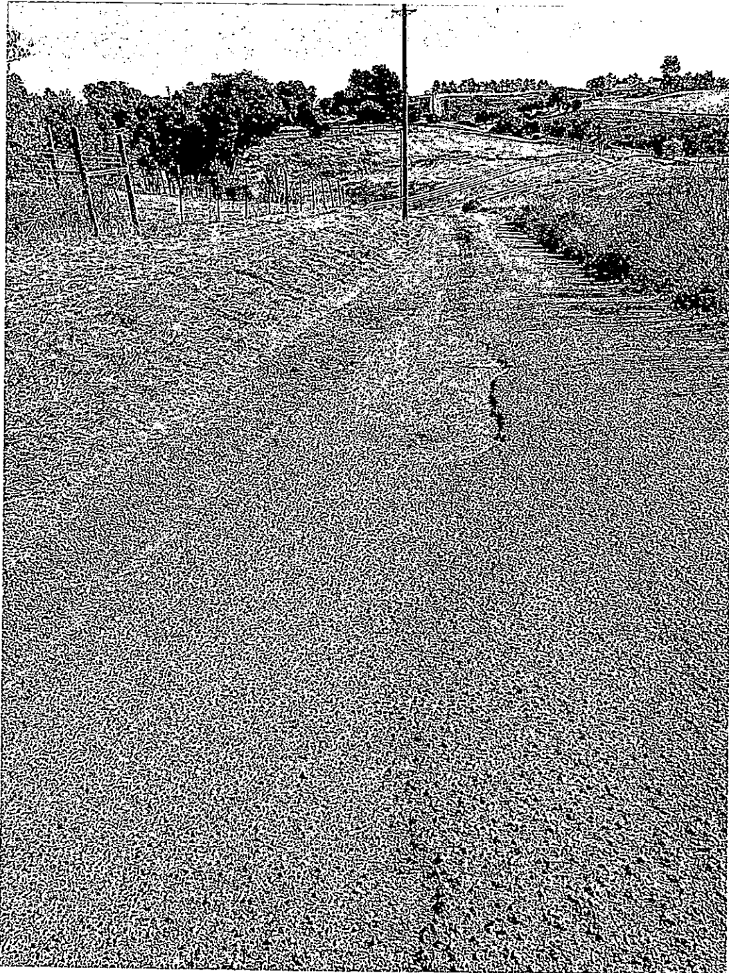
Photo 18: Independence Ranch Place, Potholes and Chip Seal Deterioration
