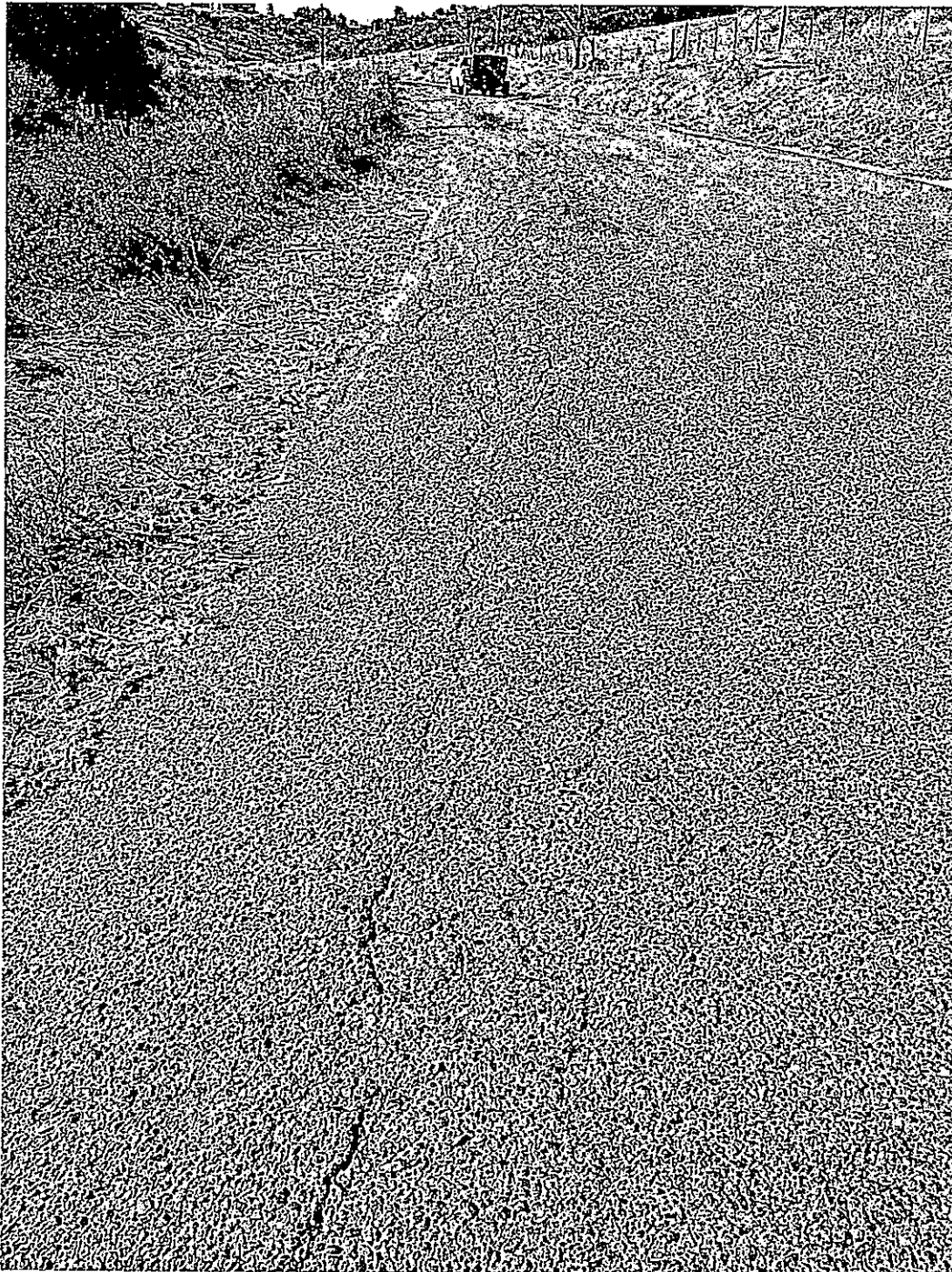
Photo 16: Hawk Ridge Place, Longitudinal Edge Cracking and Cracking in Wheel Path
