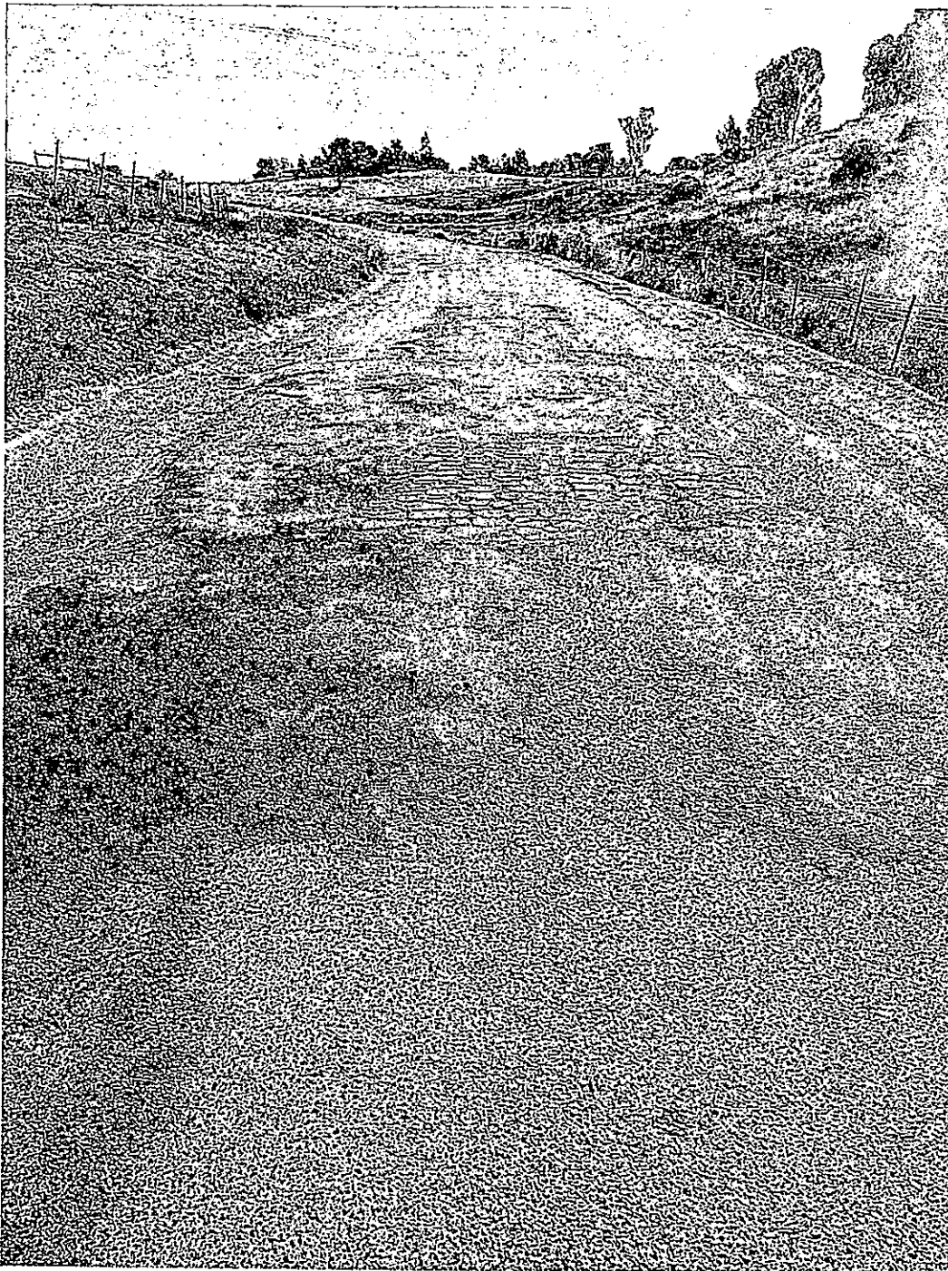
Photo 9: Avenida Trinidad Place, Shoving within Patches and Patch Deterioration
